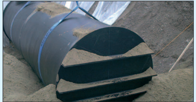
Compacted sand bed at least 500 mm thick to be provided around full perimeter
