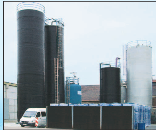
2 double-wall HDPE storage tanks, diameter 4000 mm, overall height 17,120 mm, capacity 200,000 L
